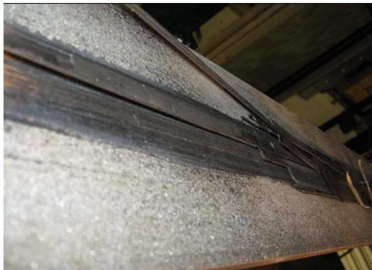
Fig. 2.43: Rupture of full width laminate
